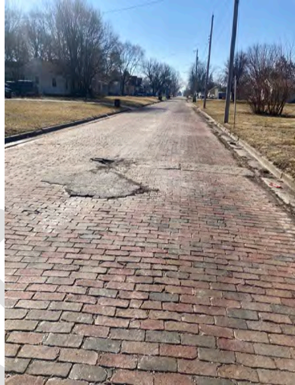
Deteriorated street right-of-way: Lombard Street
