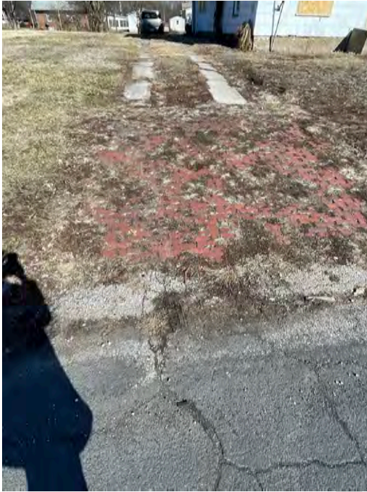
Deteriorated driveway at 1237 Mulberry Street.
